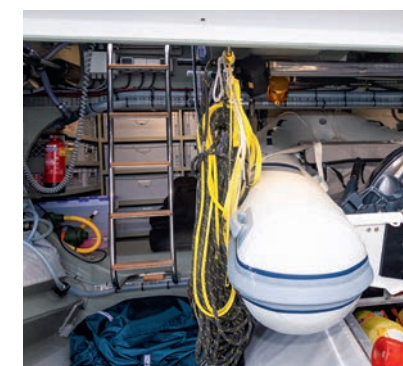
An extended stern garage allows the 2.9m RIB (modified by Contest with a folding transom) to be stored fore-and-aft for easier launching. Also back here is a fully independent bilge pump that can be used as a fire hose at the flick of two valves
